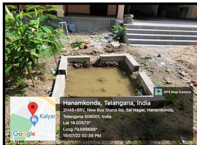
Water Harvesting pits before RUSA building
