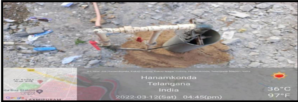
Bore well near RUSA building
